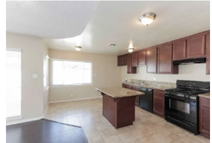
After Kitchen Remodel (no permits issued):
